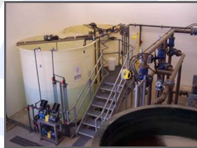
Chemical Feed System
