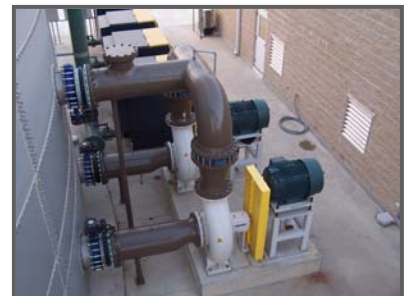
Jet Aeration System
